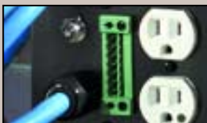
Remote control port and hospital-grade outlets
